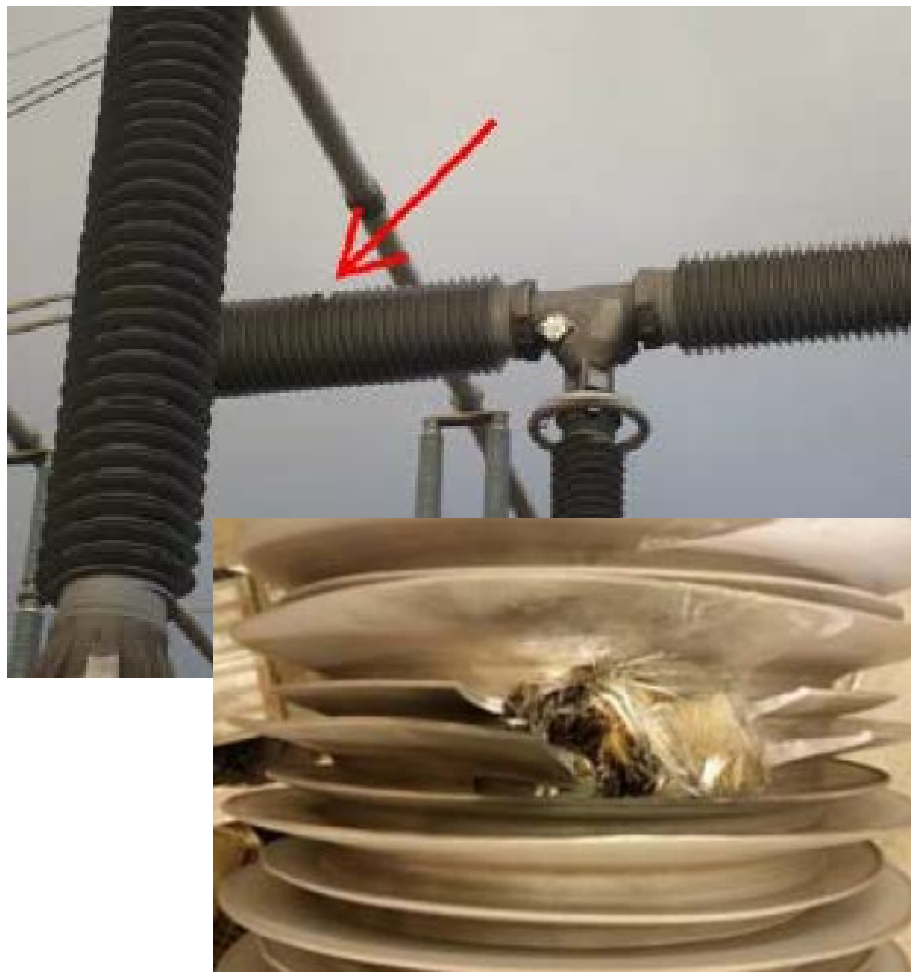
Perforation of the composite insulator.
