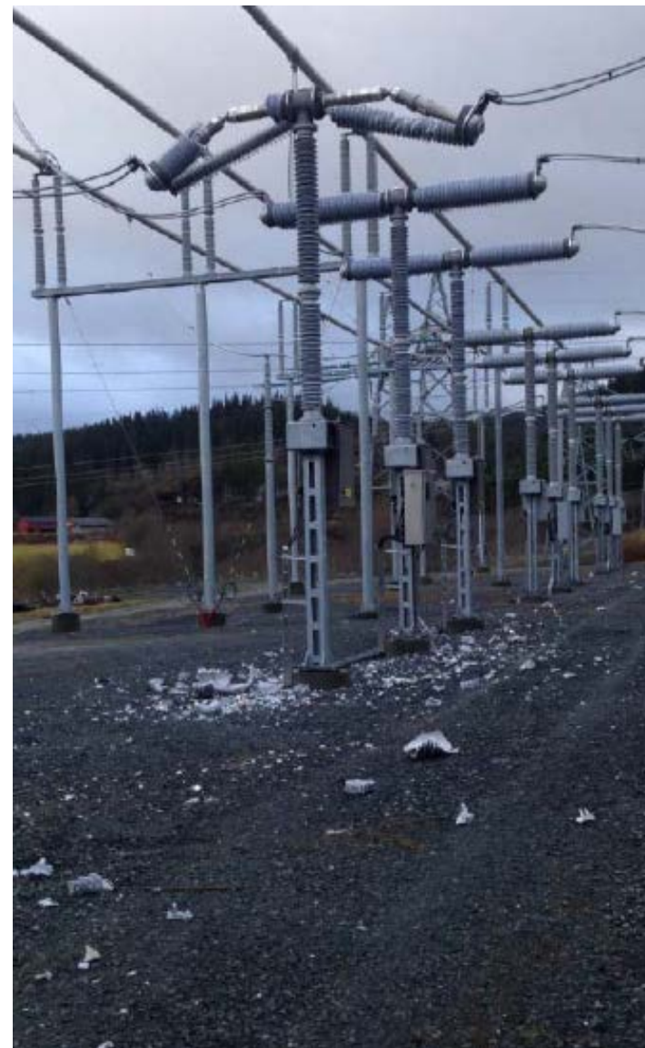
Fragmentation of 420 kV porcelain insulated circuit-breaker.
