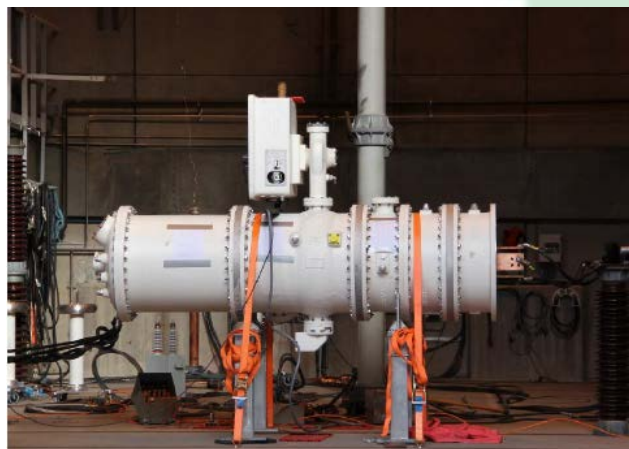
800 kV FAES assembled for making test
