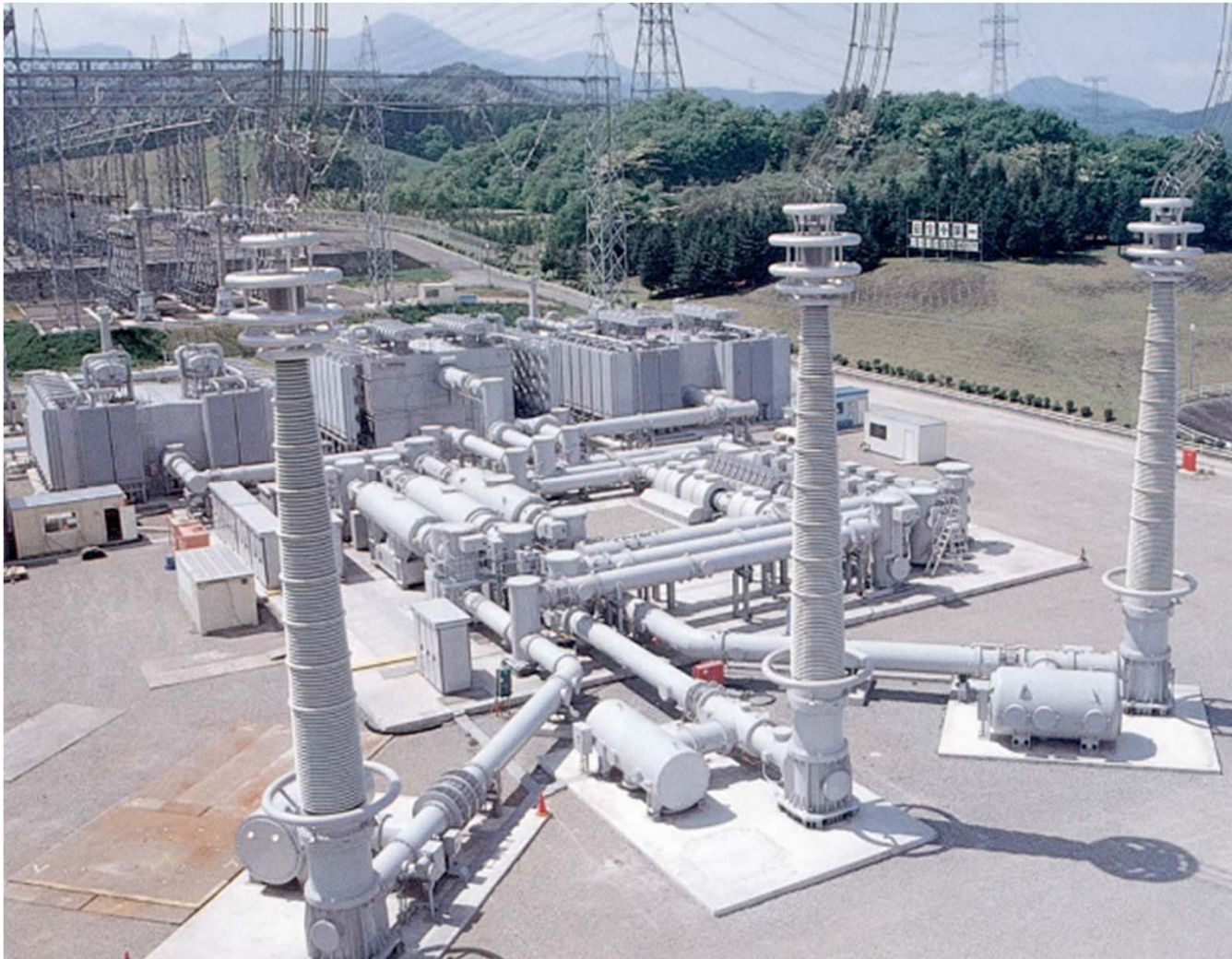
1000kV Transformer and GIS (Shin-Haruna substation : TEPCO Power Grid Inc.)
